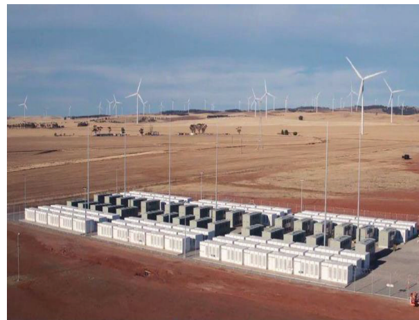
Fig.3. Large-scale battery storage system [31]
